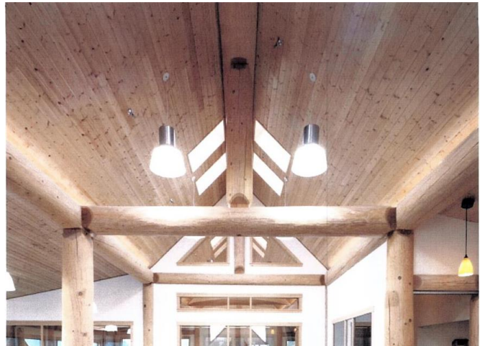
Quilakwa Center ceiling — Featuring locally sourced wood. Photographer, Peter Sperlich. Photo courtesy of Wood Design & Building Awards.
