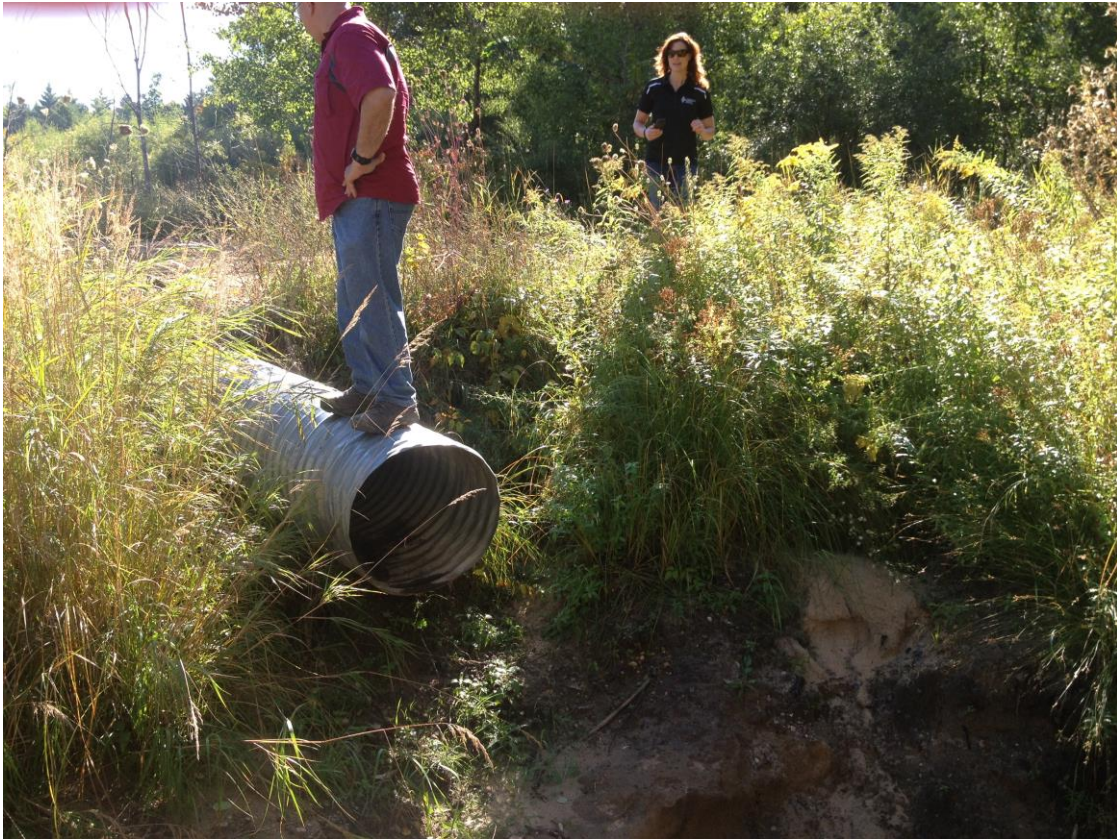
Auditors examining badly perched culvert.
